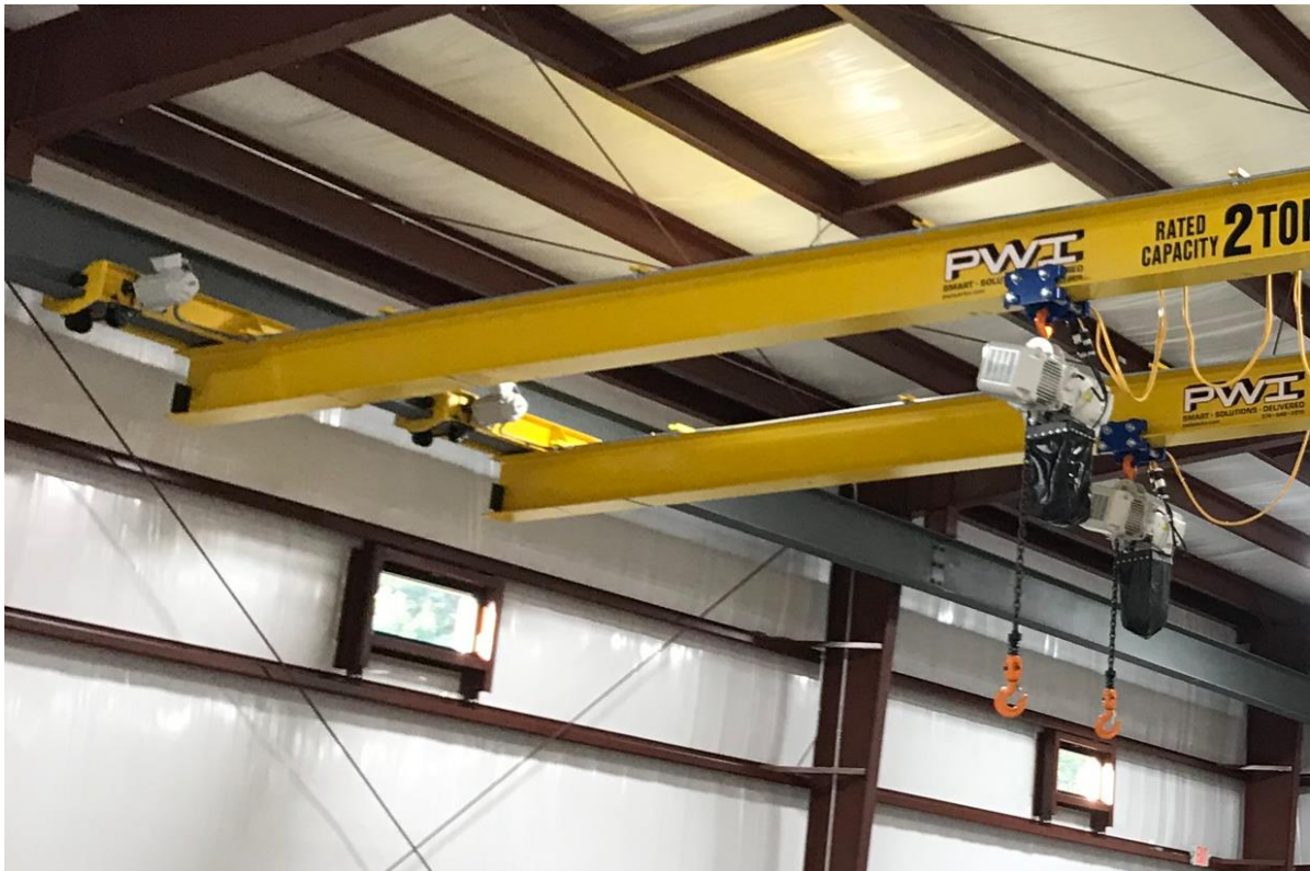
1.1 SCU Under-Running End Truck
