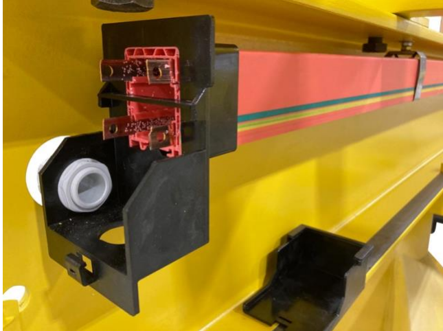
4.6.1 End of ElectroTrack System
