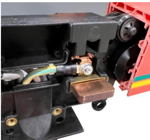
4.6.9 40 Amp Single Collector Installed
