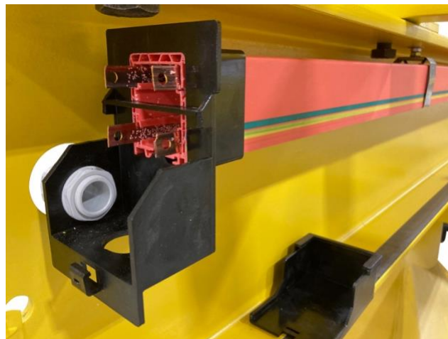
2.3.1 End of ElectroTrack System
